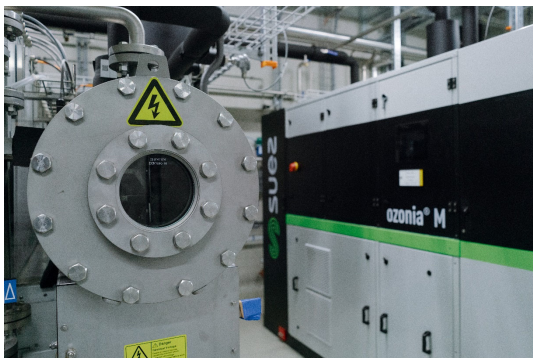
Foto: Ozongenerator ARA Altenrhein, by Milad i.A. VSA
